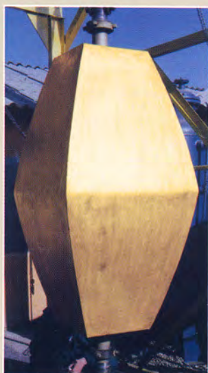
LEFT: A SEGMENT OF THE ENDLESS COLUMN DURING THE RESTORATION PROCESS. ABOVE: A RESTORED SEGMENT AFTER FINAL REPLATING.
