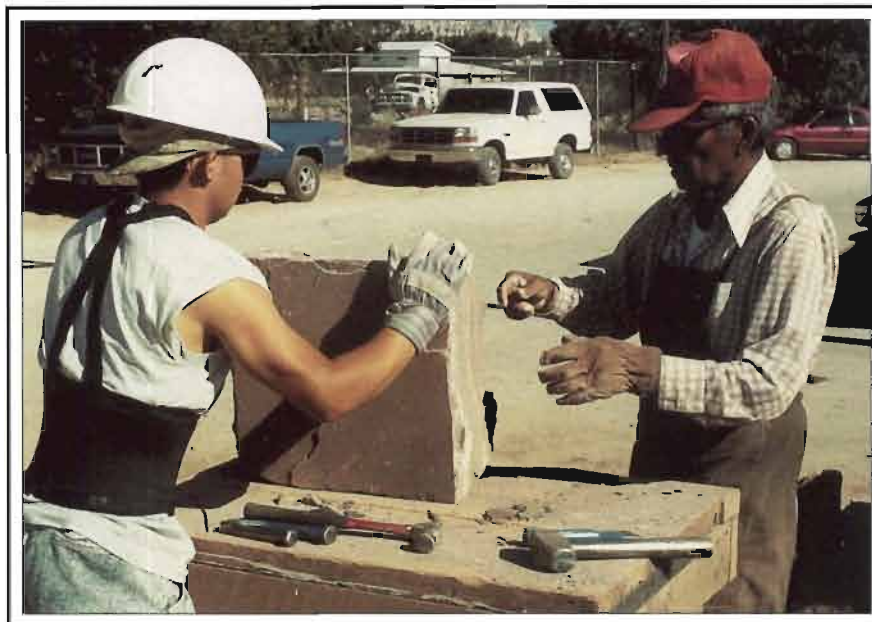
AT ZUNI PUEBLO, NEW MEXICO, A TRIBAL ELDER INSTRUCTS YOUNG MASON ON PROPER STONE DRESSING PROCEDURES
