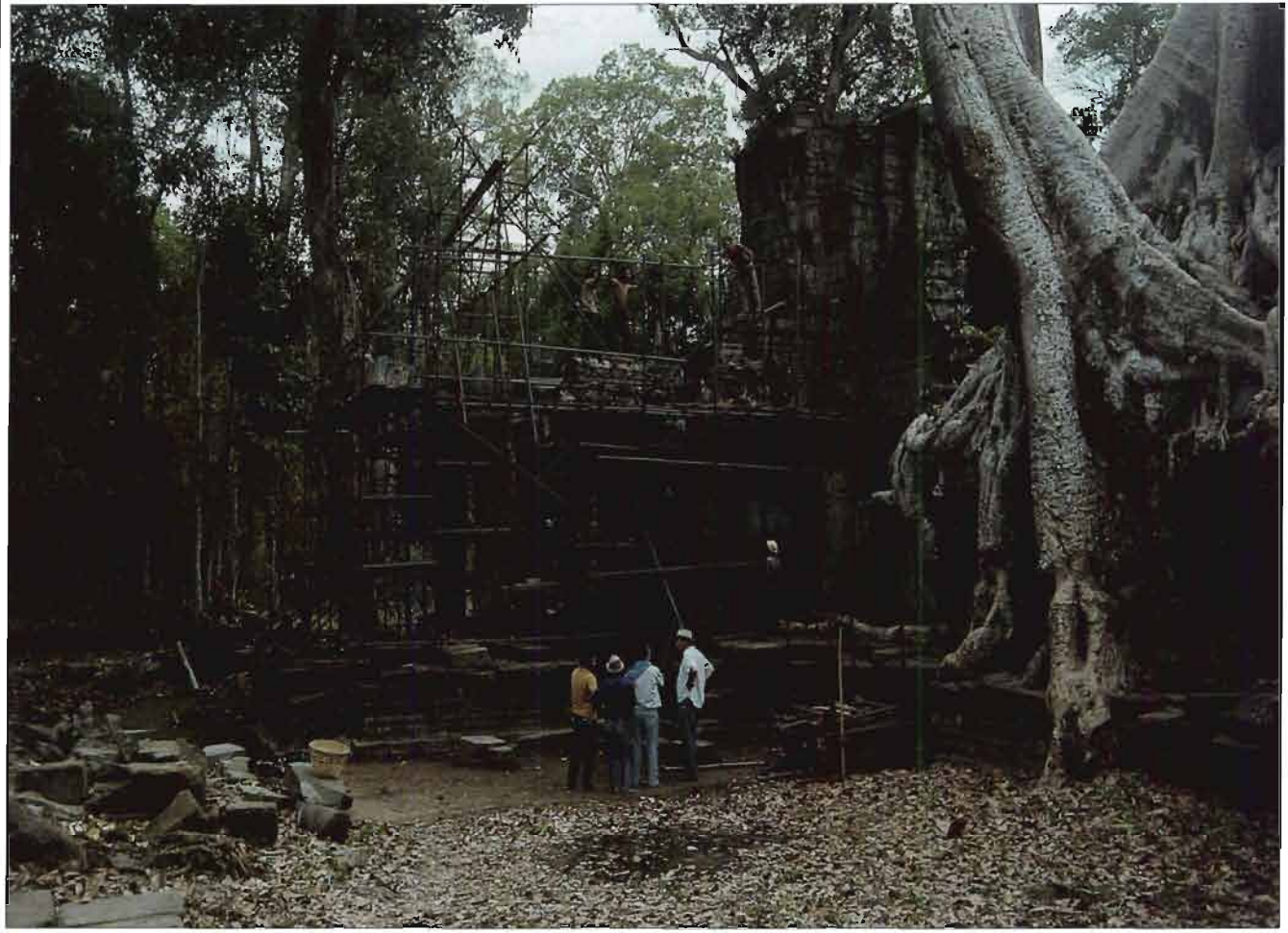
PREAH KHAN TEMPLE COMPLEX, HISTORIC CITY OF ANGKOR, CAMBODIA: WMF FIELD TEAM MONITORING STRUCTURAL STABILIZATION AT THE SOUTH PORTICO OF THE EAST GOPURA (ENTRANCE GATEWAY)
