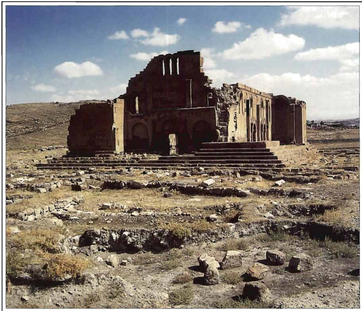
TOP LEFT: DETAIL OF APSE TOP RIGHT: EMERGENCY STRUCTURAL SHORING ERECTED BY WMF TEAM ABOVE: OVERALL VIEW OF THE EREROUK BASILICA
