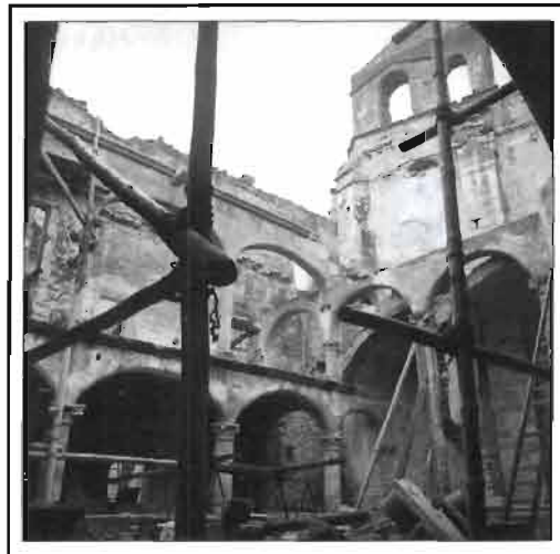
TOP: DETAIL OF THE PATIO AFTER RESTORATION ABOVE: ARCADED PATIO BEFORE RESTORATION OPPOSITE: A MEETING ROOM. AFTER RESTORATION
