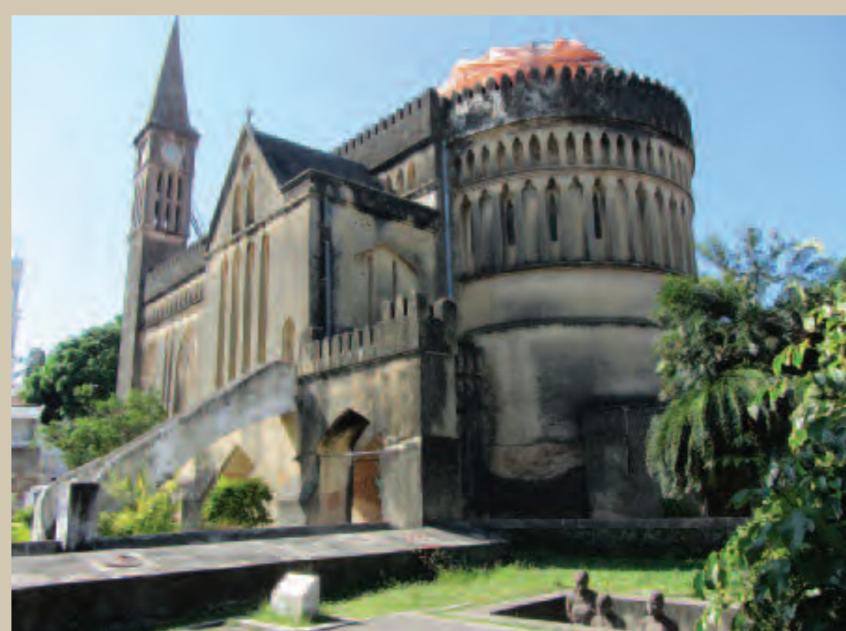
The deteriorating condition of the cathedral before the start of the project, pictured in 2013 with plastic sheeting on the roof providing temporary protection.
