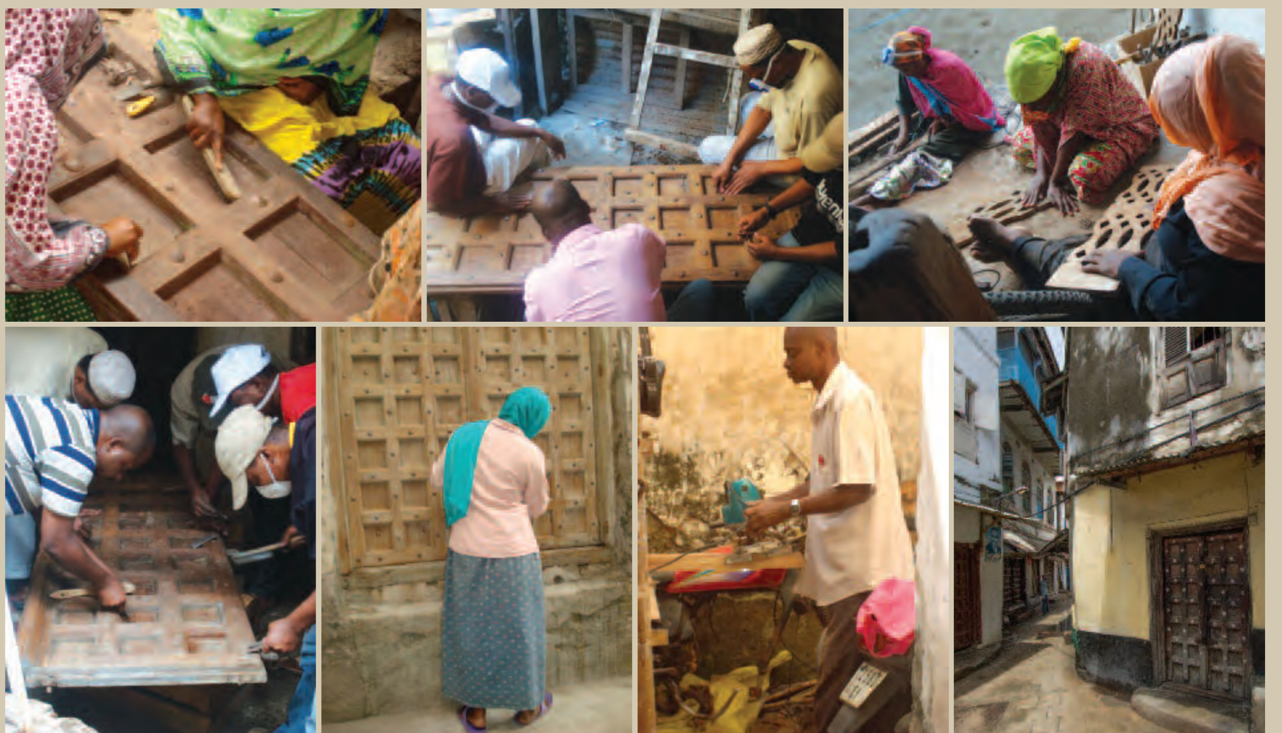
Timber conservation training: the practical component of the course took place at a house in Stone Town, and was implemented by Zanzibar Stone Town Heritage Society. The training involved instruction by a skilled carpenter in the repair of doors, windows, a balcony and staircase.
