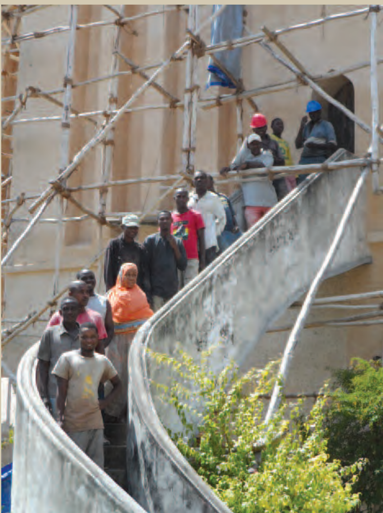
Conservation was led by a master stone mason alongside a skilled team of local craftspeople.
