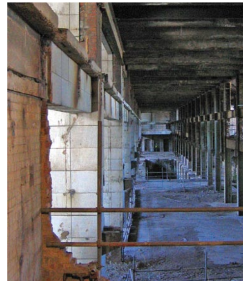
THOUGH DILAPIDATED, BATTERSEA'S ENORMOUS ART-DECO INTERIORS STILL BOAST DETAILS LIKE SIR GILES GILBERT SCOTT'S ORIGINAL MARBLE WALLS AND COLUMNS.
